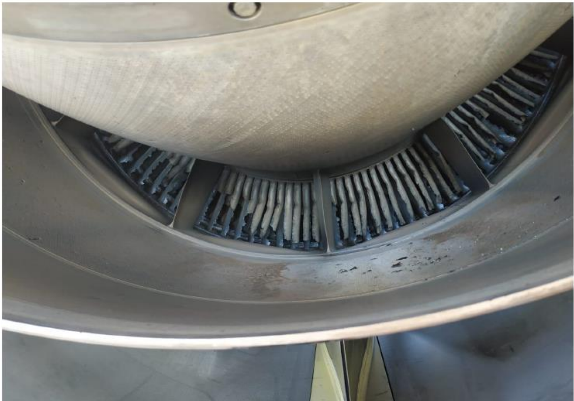
Picture 3: external evidence of left engine damage.
