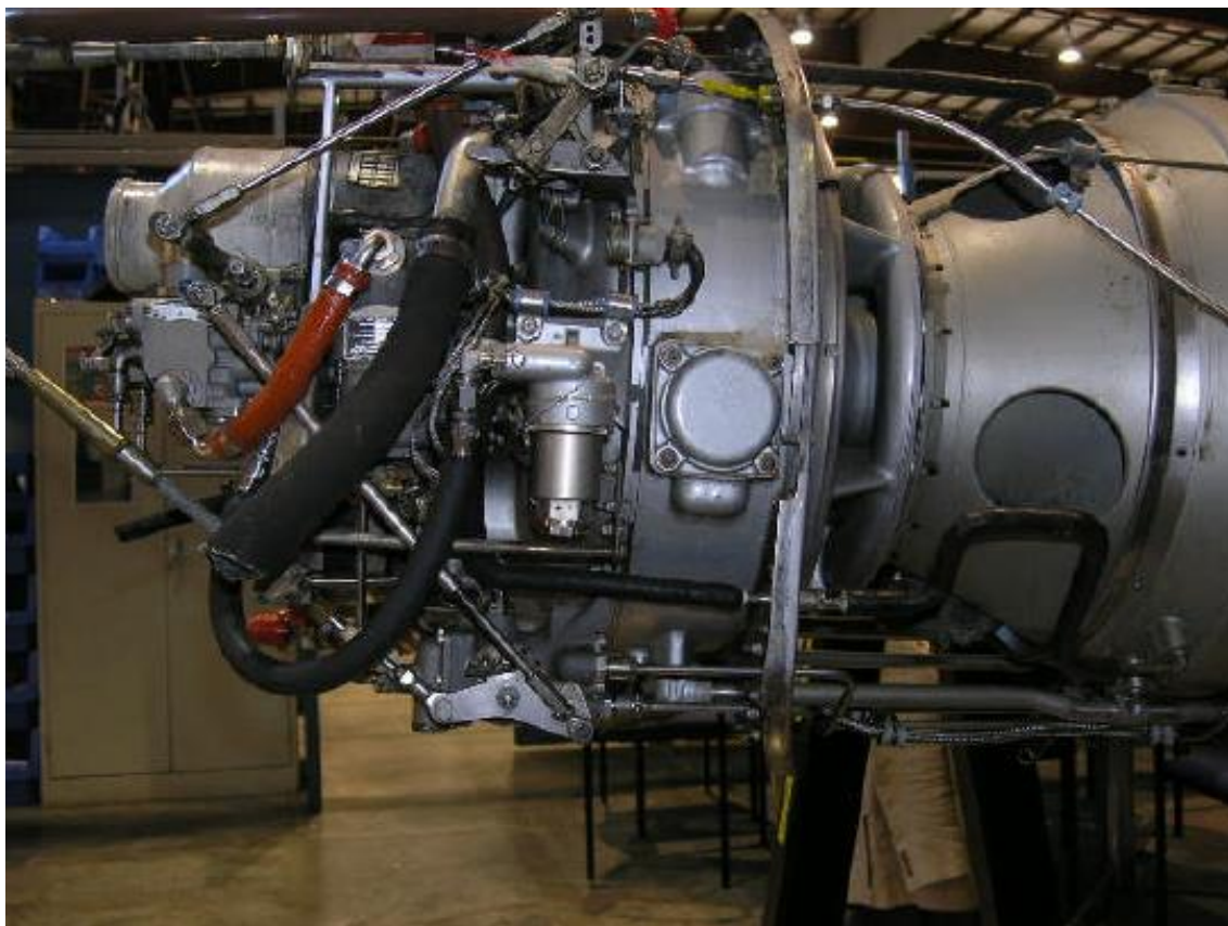
Foto 13: gas generator case e accessory section.
