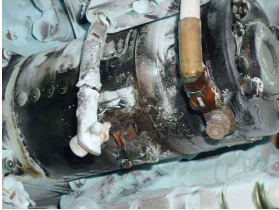
Picture 1: electrical connectors and cable as found after fire extinguished.
