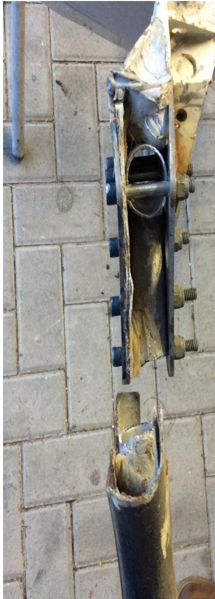
Photo 12: ovalisation of the tubular rib due to the pressure of the bolted plates.
