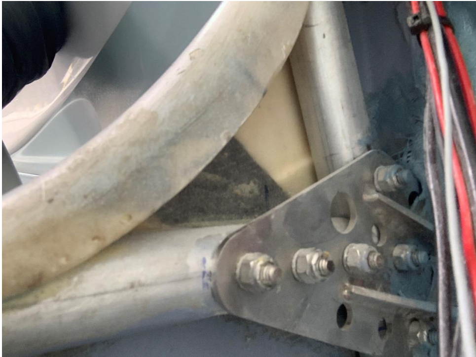
Photo 5: rear view of the metal plate constraining the wing strut and the structure's aluminium tubulars (right wing strut fixing point). Photo taken during the ANSV inspection of an aircraft of the same type the one that crashed, on the "Leonardo da Vinci" airfield in Vigevano.
